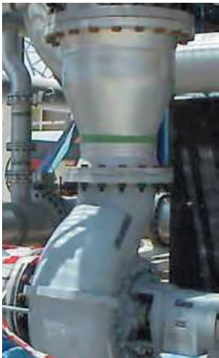
Cooling water pump for primary turbine at a power plant in the Middle East.
