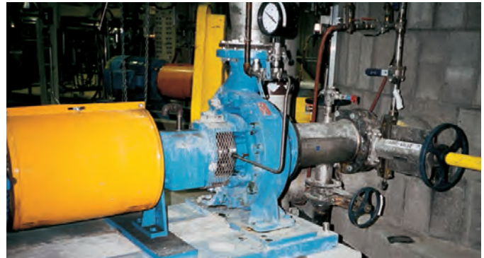
Installation at a North American recycle mill.
